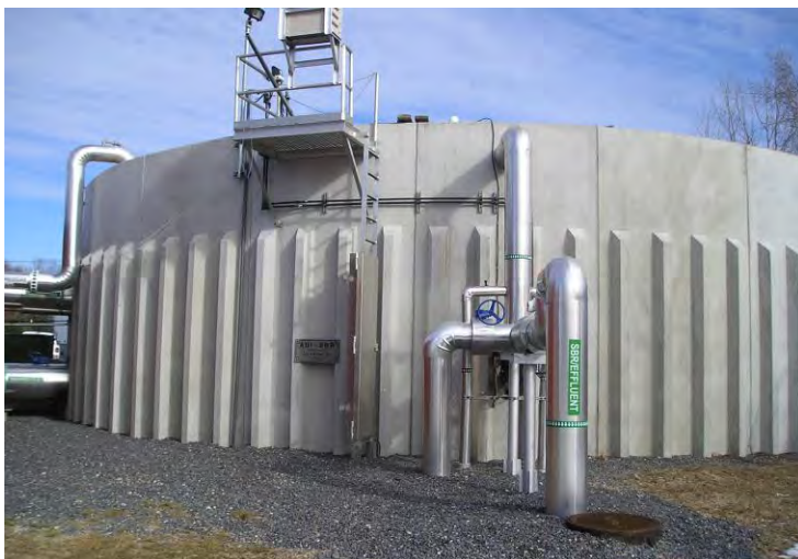
2.3 MG SBR tank installed by Dutchland for Ken's Foods in 2000
