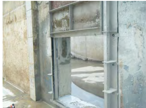
Installed sluice gate.
